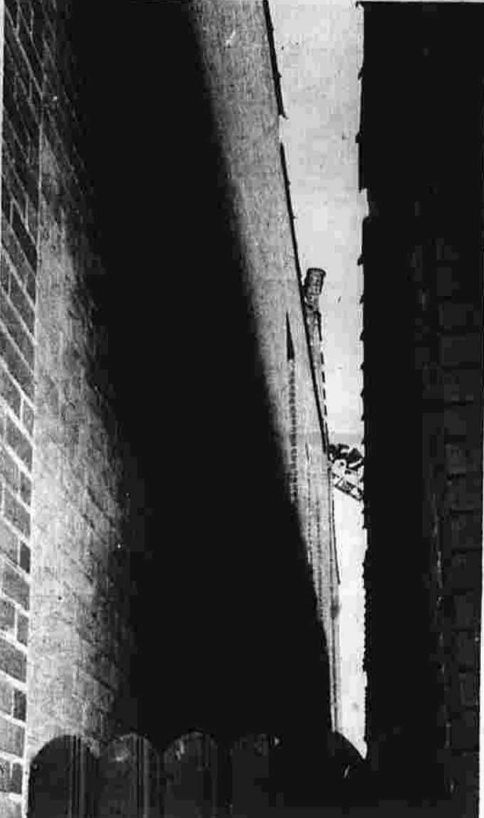
Nervous moments A brick parapet on a building on 745 Main St. pitches precariously as members of the Town of Manchester Fire Department climb onto the roof of the building to check it out Thursday afternoon. Tenants of the building were evacuated Thursday afternoon. The picture was taken looking through a small alley between two buildings. (Herald photo by Richmond)
